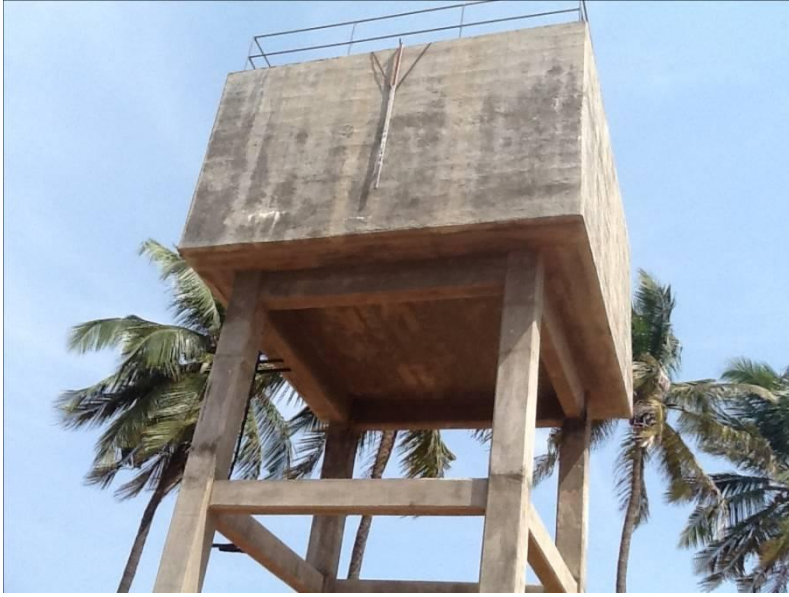
Water Supply System
